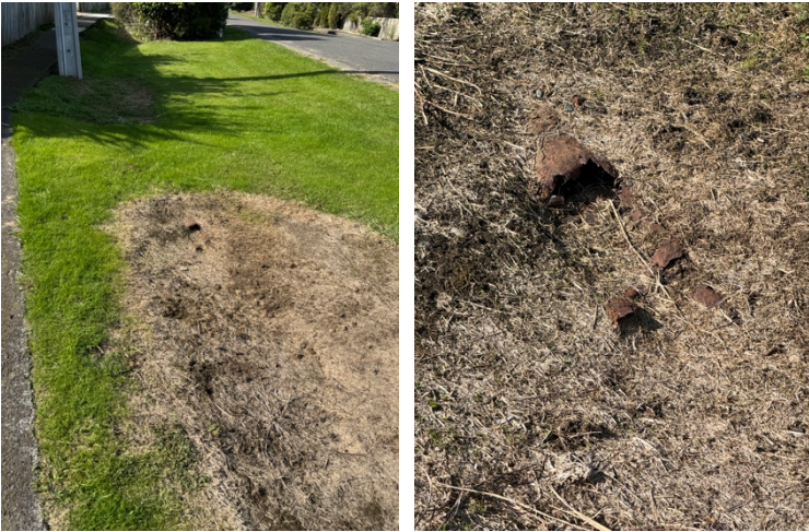
This is an exposed culvet pipe – just waiting for some poor child to cut their foot on, or anyone that slips down due to the uneven footpath and cut themselves.
