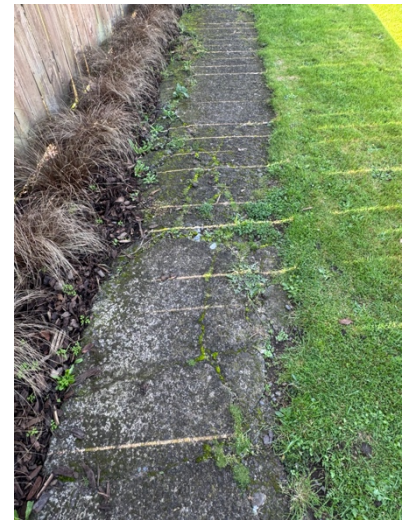
Whilst some parts have been patched up – others sections are in a shocking state!
