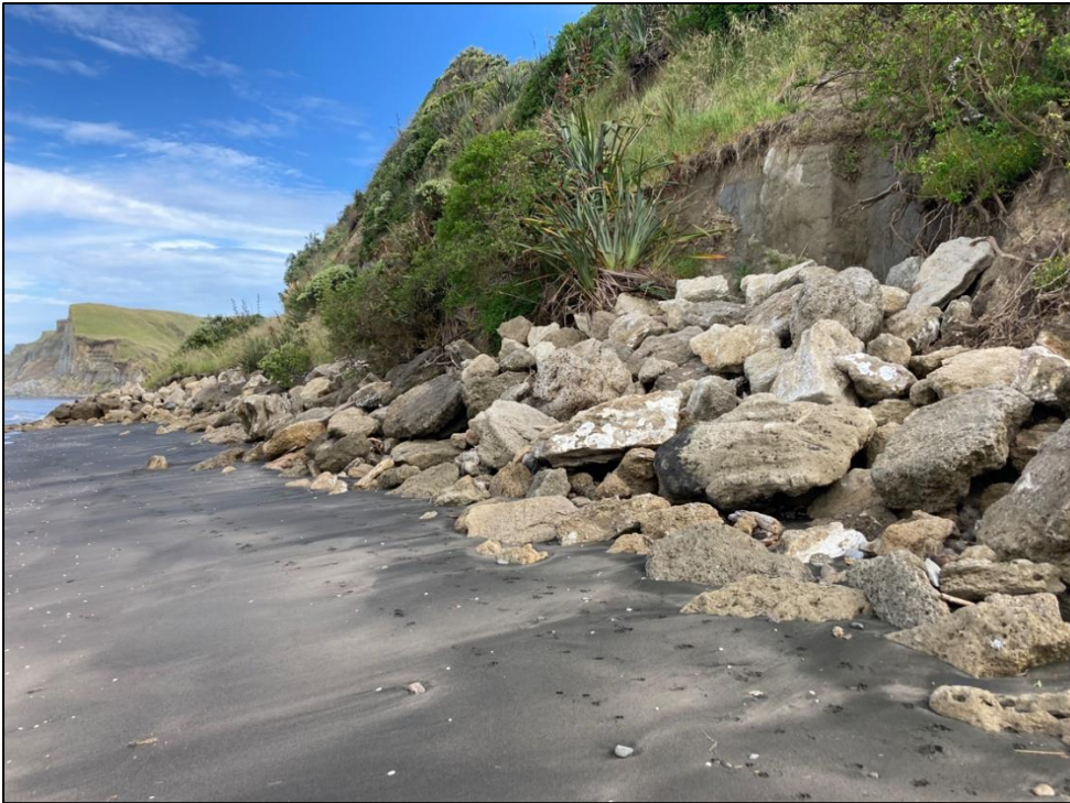
Photograph 3.5: Existing 'shell rock' revetment between the Kai Iwi and Mowhanau stream mouths
