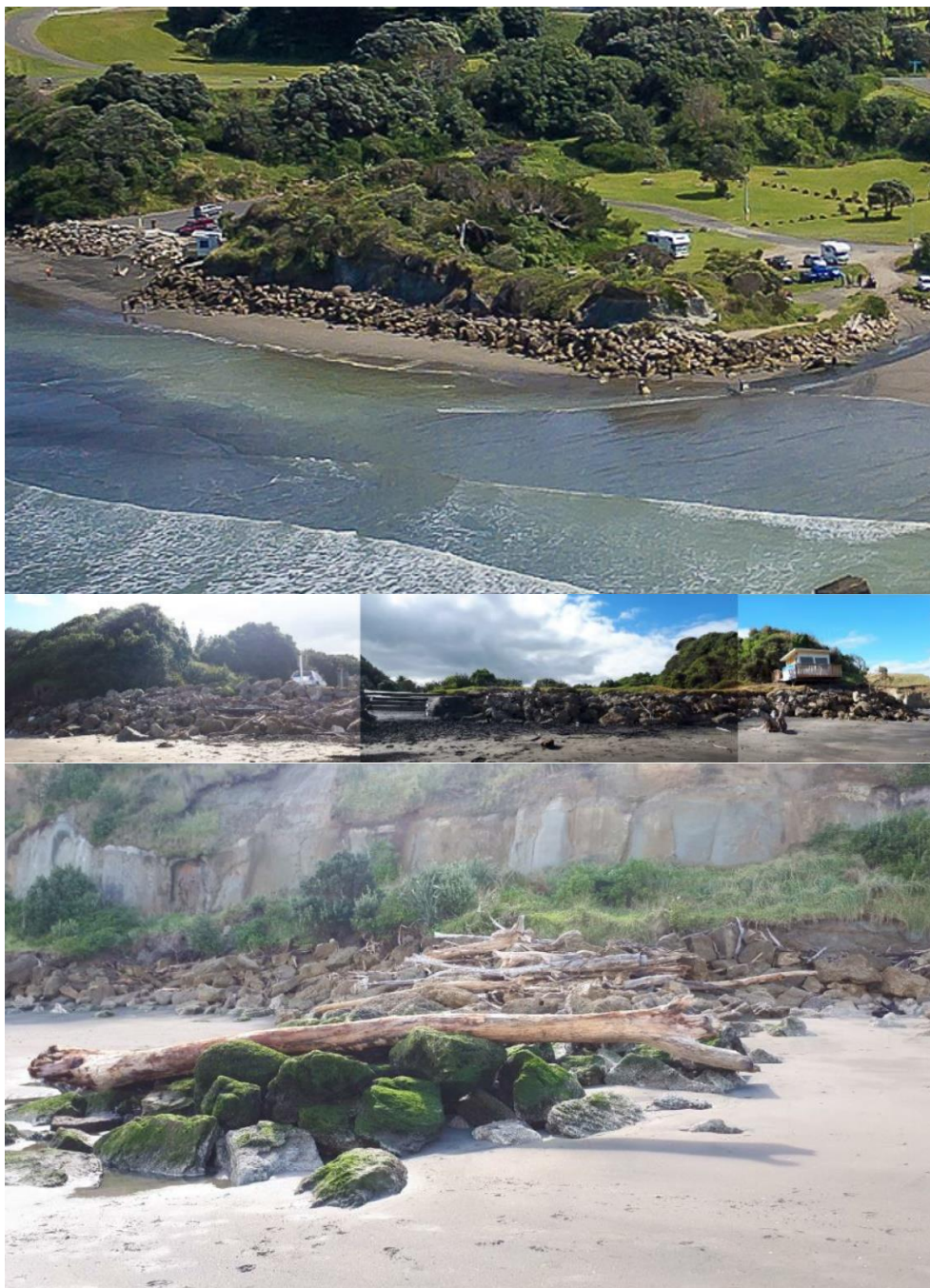
Photograph 2.4: Existing 'shellrock' revetment running along the toe of the cliff at Kai Iwi Beach and smaller groyne within the revetment (source: Top – WDC, 2022, Middle and Lower – eCoast, 2020)
