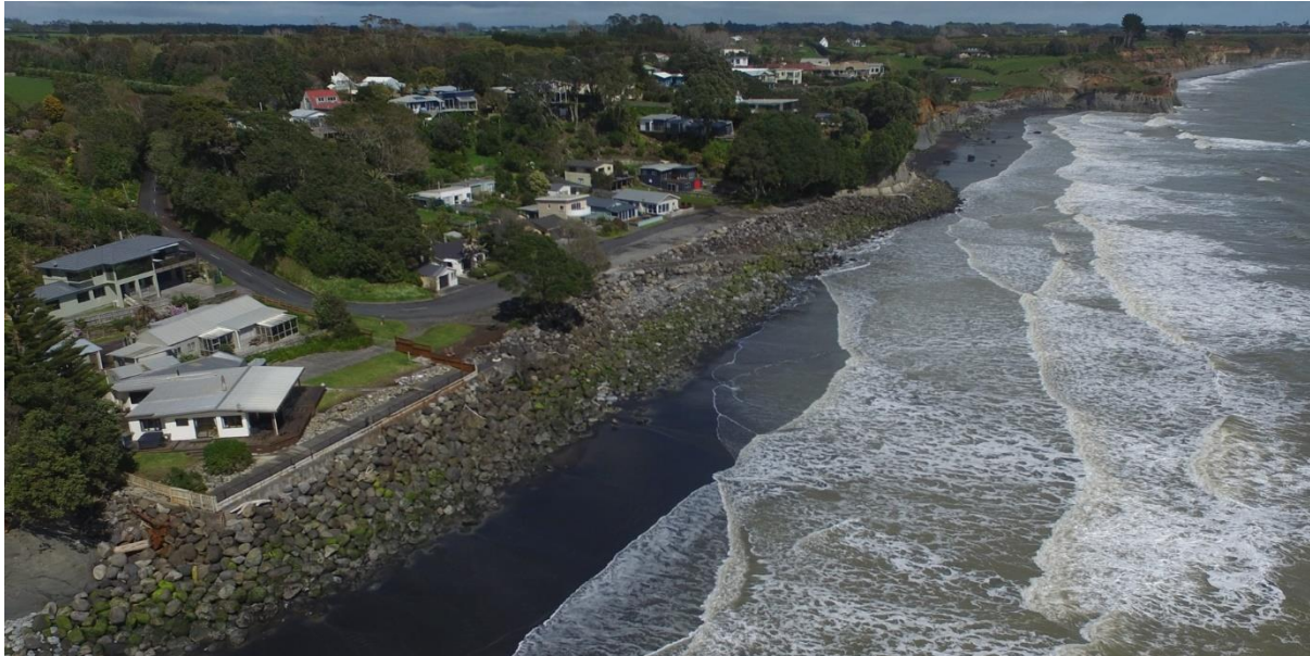
Photograph 3.6: Example of a rock revetment along the cliff shoreline at Onaero, Taranaki protecting a low backshore and carpark in the foreground and cliff headland in the middle of the beach while the cliff adjacent to the wall (top of photo) continues to retreat
