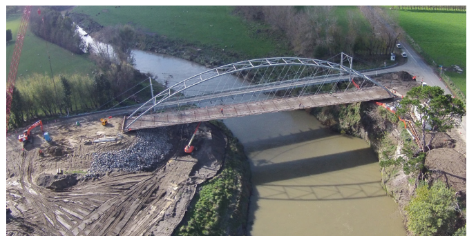
Top: Members of the Wyley family cross the bridge. Bottom: An aerial shot of the Wyley's Bridge build (May 2015)
