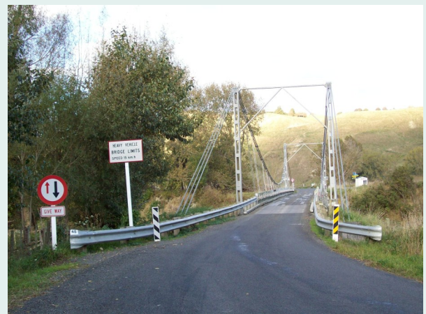
Wyley's Bridge, which Mangamahu residents use to get in and out of their community. The community has supported maintenance work with a $200,000 contribution.
