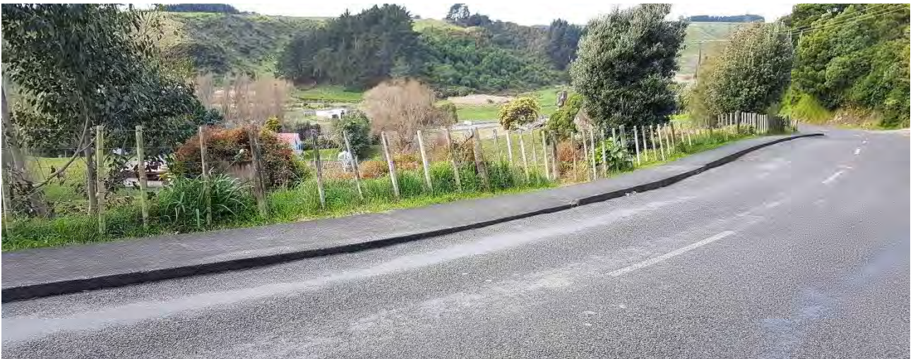
Illustration 5-1 : Minor deformation of pavement on Marybank Road
