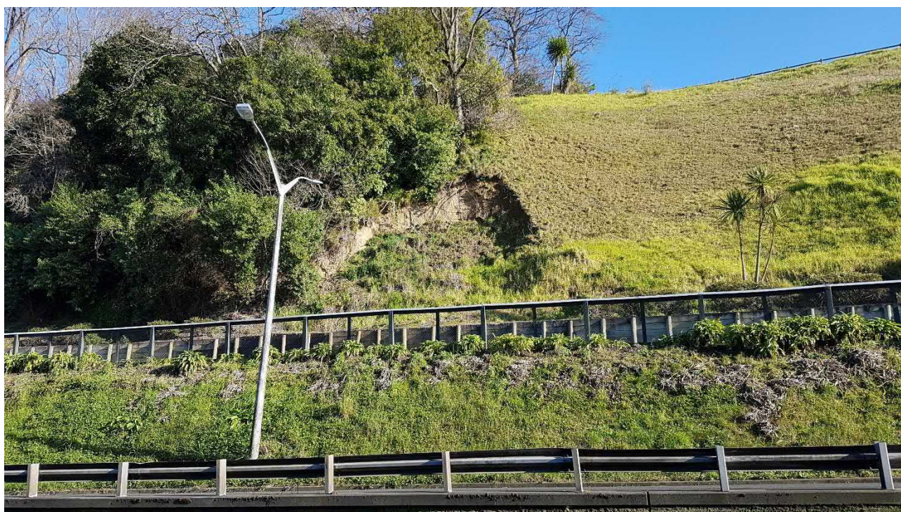
Illustration 5-3 : Landslide on steep slope
