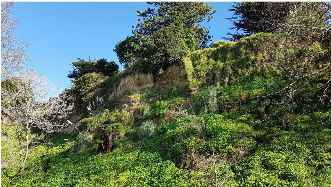
Illustration 5-4 : Slump of siltstone at crest of steep bluff
