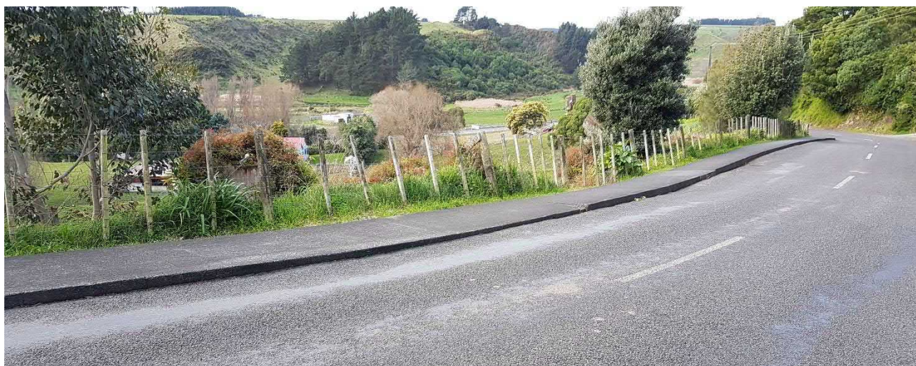
Illustration 5-1 : Minor deformation of pavement on Marybank Road
