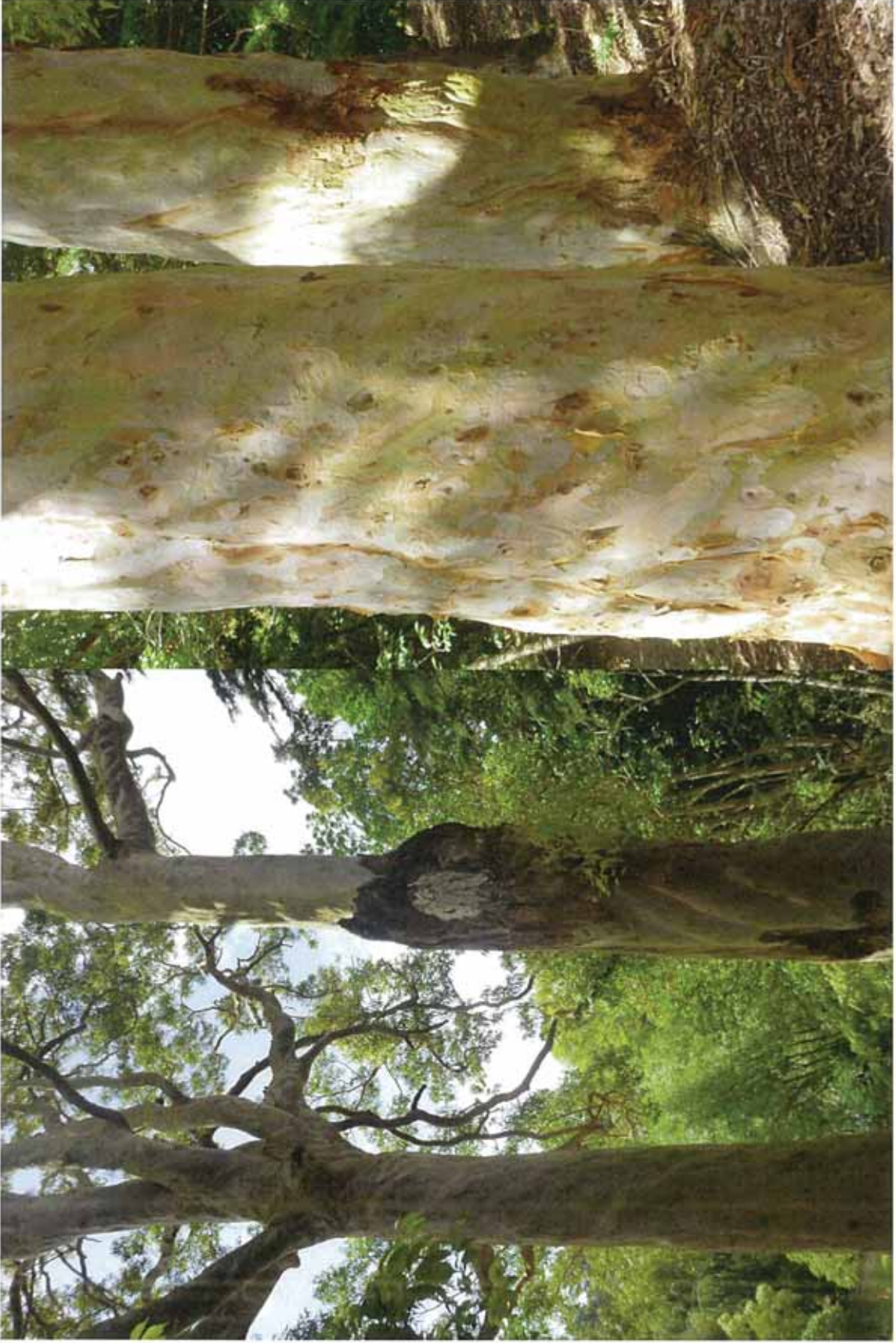
Large failure in tree (not included in assessment) next to well-formed tree.
