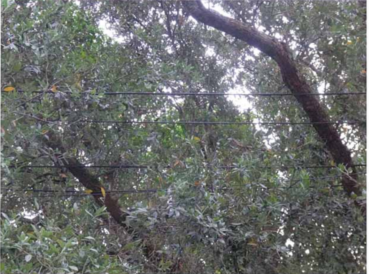
400v power lines rubbing on large branches.
