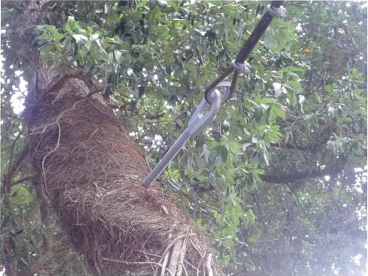
Steel bracing attachment into Pohutukawa leader.
