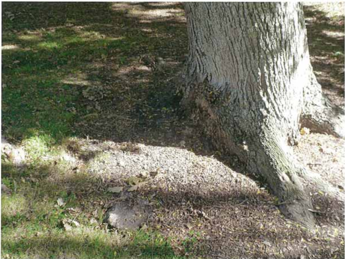
Tree 2 showing removed/failed trunk.
