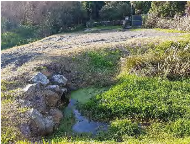
C: One of the many existing culverts conveying the unnamed stream under private accessways.
