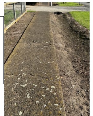
Footpath has a huge high lip, that then falls down into an open drain
