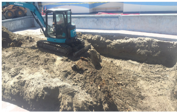
A contractor prepares to remove large tree roots found underneath the floor of the Whanganui East Pool
