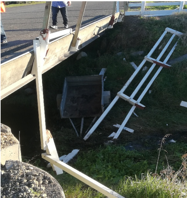
Photo 2: Damaged bridge on No. 3 Line over the Matarawa Stream following recent crash
