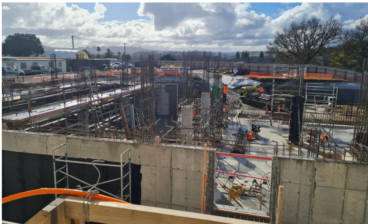
Figure 3. Construction of the three story extension wing in progress showing basement construction and the start of installation of formwork for the next level floor.
