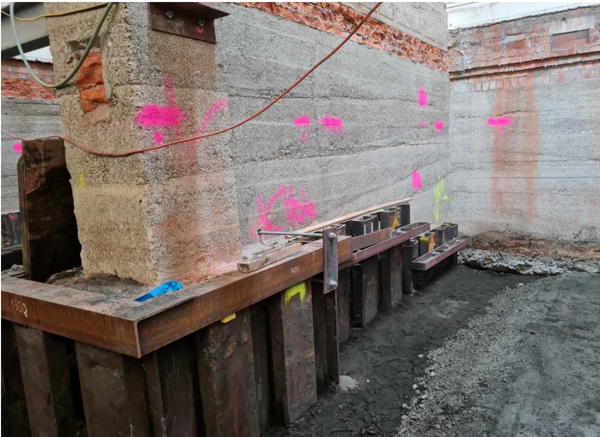
Figure 1. East wing where sheet piles have been installed to support the existing foundations.
