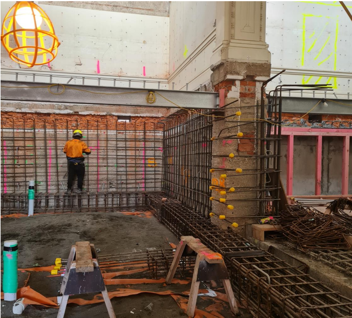
Figure 2. West wing where workers are tying reinforcing against the existing old basement walls before concrete is poured, with some of the new concrete walls visible to the right.
