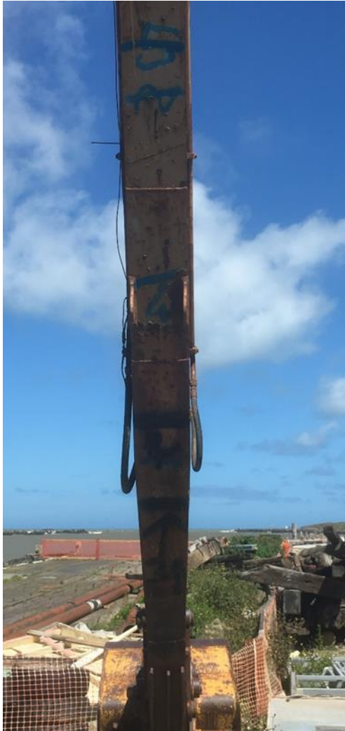
Figure 8. The depth to which an area is dredged has been previously gauged by a painted scale on the arm of an excavator operated from a barge or wharf.
